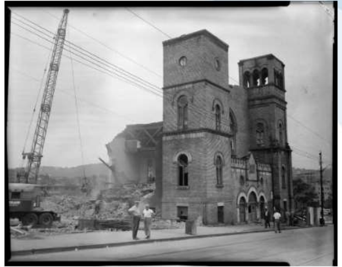
"Demolition of Bethel AME Church, Wylie Avenue and Elm Street, Lower Hill District, Pittsburgh, Pennsylvania, July 24, 1957." (Photo by Charles 'Teenie' Harris/Carnegie Museum of Art/Getty Images)
