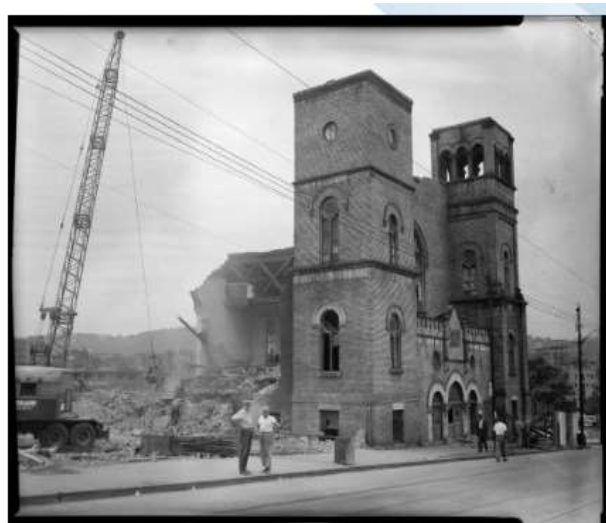
"Demolition of Bethel AME Church, Wylie Avenue and Elm Street, Lower Hill District, Pittsburgh, Pennsylvania, July 24, 1957." (Photo by Charles 'Teenie' Harris/Carnegie Museum of Art/Getty Images)
